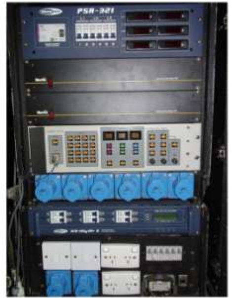
Above: 32amp 3-Phase distribution rack
