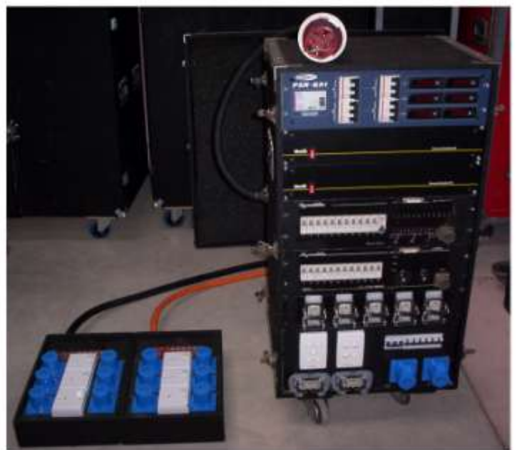
Above: 63amp 3-phase distribution rack.
